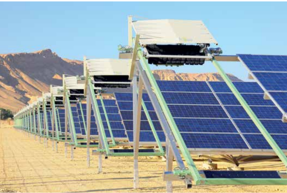
Ecoppia E4 robots in their docking stations, waiting for the sun to go down.
