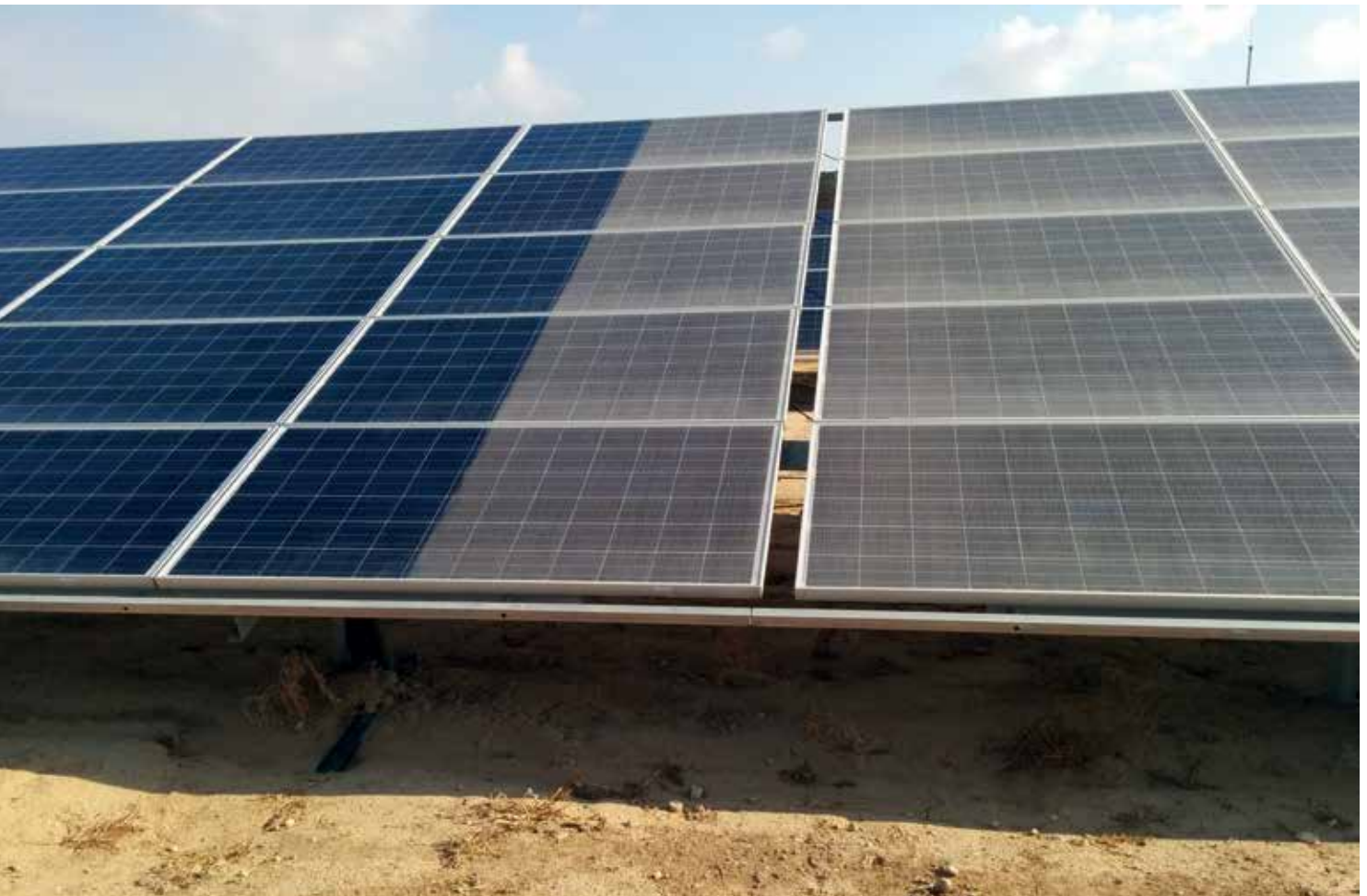
Side-by-side comparison of panels maintained by Ecoppia's E4 and those seeing intermittent manual cleaning.
