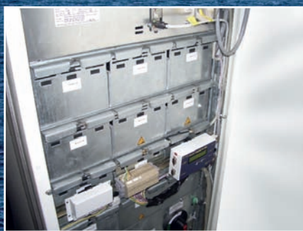
Battery analysis and care system
